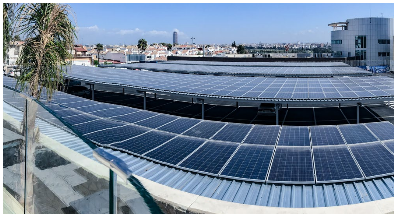
Photovoltaikanlage Gran Casino in Sevilla
